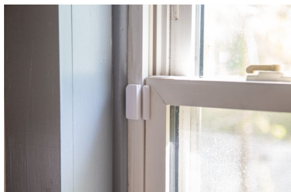
Picture 39 – Open/Close Alarm Sensor for SCW Shield - 74WOS
